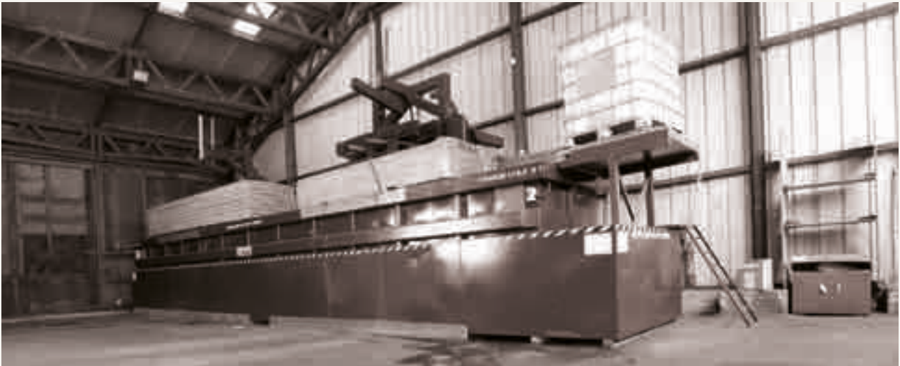
Class 2 treatment tank - Bouguenais site (44)
